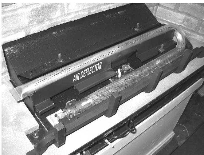
Figure 25. Correct burner tube alignment.
